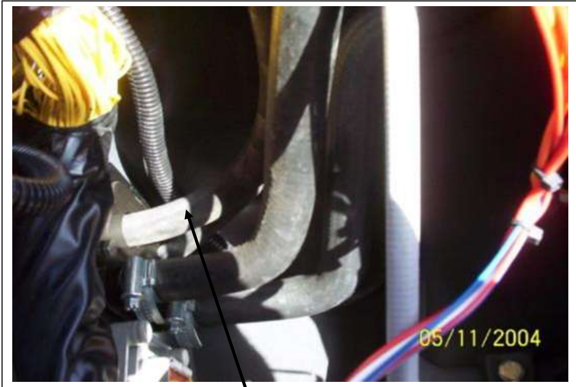
A/C lines running up to the evaporator coil
