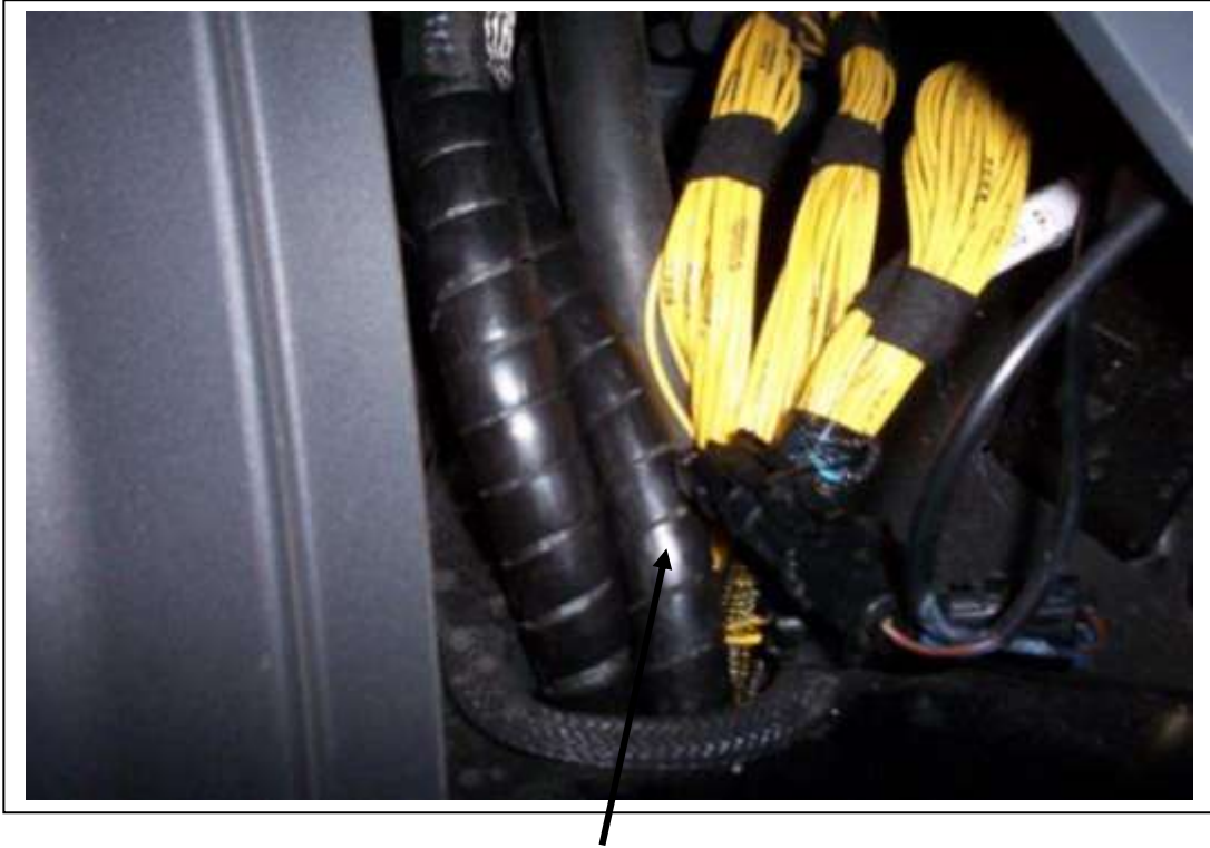
A/C hoses and clutch wire coming up through the floor to the left of the fuse panel
